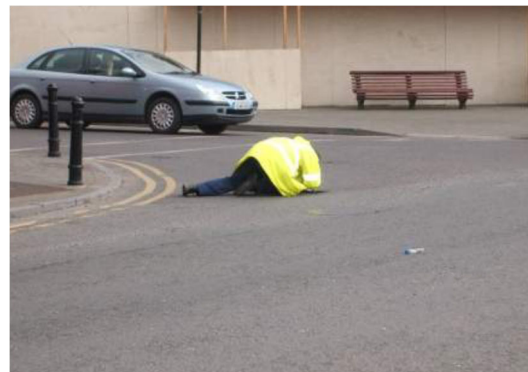
Figure 0.2.2.2.2: An unprotected road worker working in a live lane is not Type C Works
